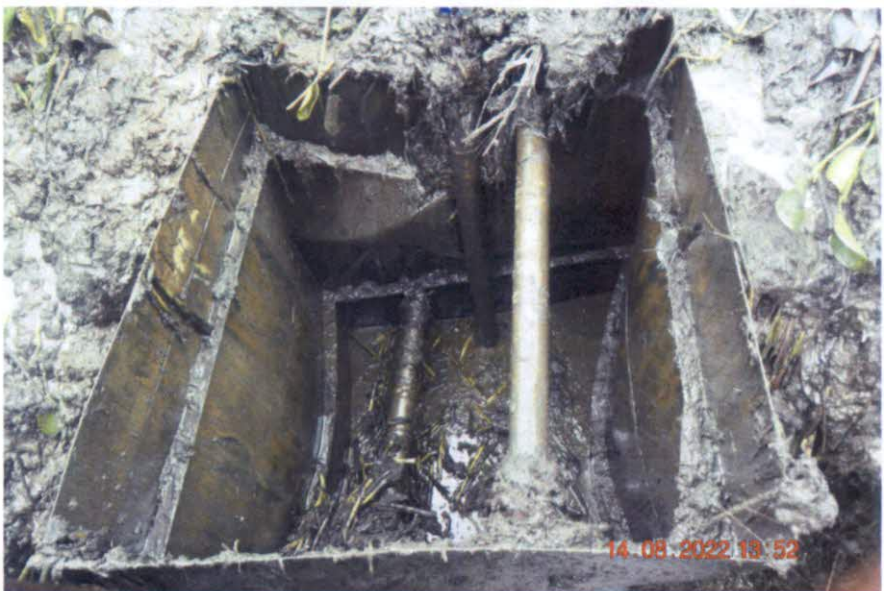
Fig. 3 The 4" Ball valve attached to the 16" for Oil Theft
