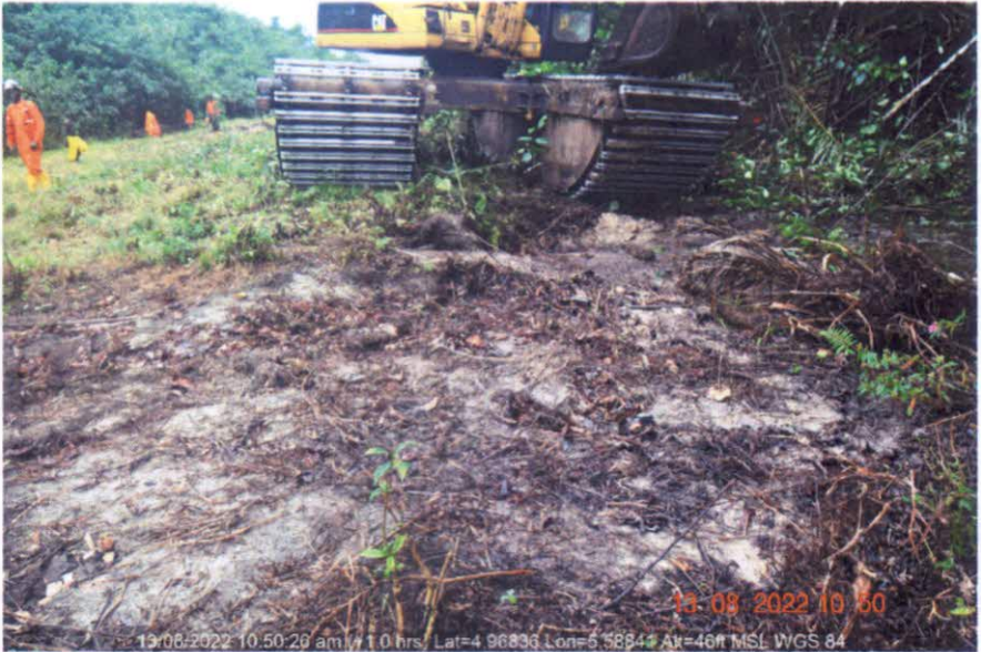
Fig. 1 Incident Area on Arrival of the JIV
